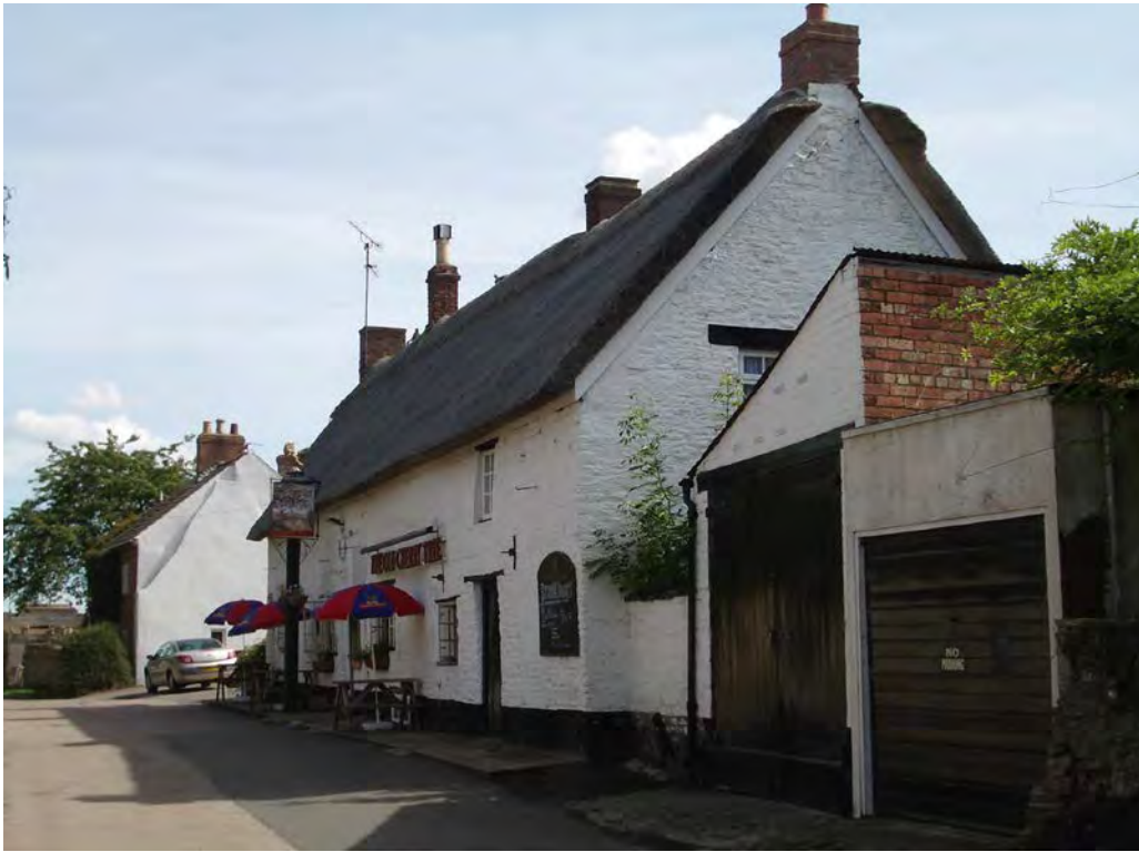
The Old Cherry Tree Inn - reed thatch replaced a corrugated iron roof
